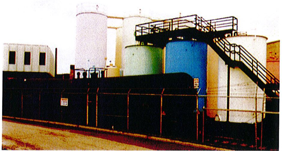
Products are delivered to Houghton Chemical's 450,000-gallon bulk plant next to its offices in Boston by rail tankcar and tank trailers. The bulk plant has six railcar spots, which are heavily used.
